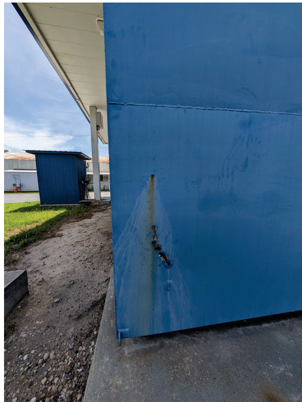
Exhibit 1-20: Fuel Storage Tank
